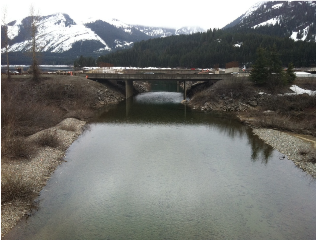
Photograph 2-1 View facing west of the eastbound Gold Creek Bridge, beyond which is Keechelus Lake. May 2011.
