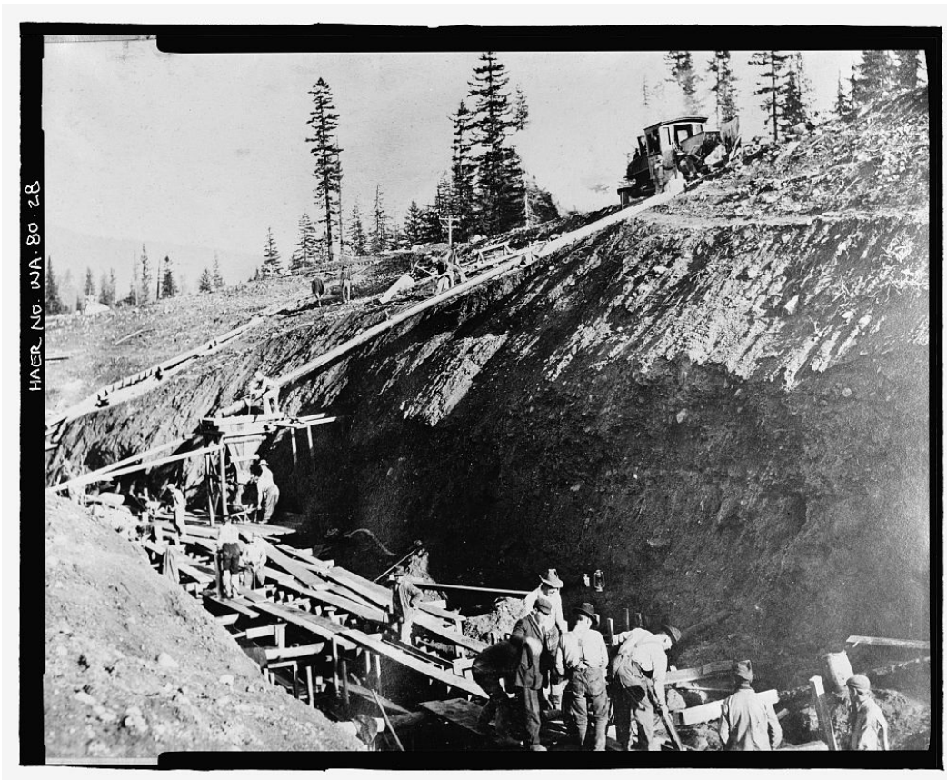
Photograph 3-15 Keechelus Dam Construction, October 1913. Placing concrete in core-wall from concrete cars operating on the trestle. This image also illustrates the size and scope of the support facilities needed to construct the project (USLC, HABS/HAER).
