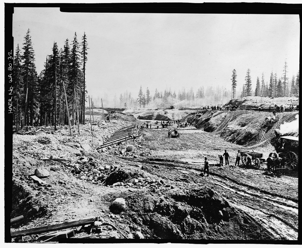
Photograph 3-12 Keechelus Dam Construction, June 1914 Building the embankment; A section of the foundation and riprap rock in place is shown on the left (USLC, HABS/HAER).
