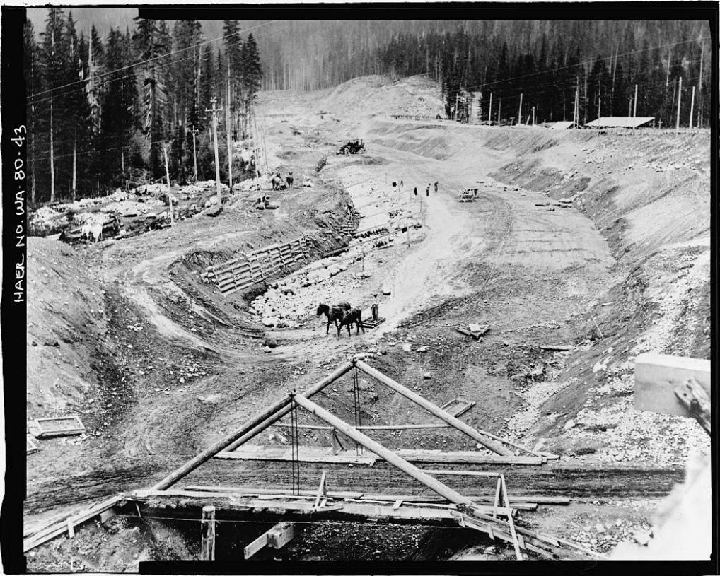
Photograph 3-14 Keechelus Dam Construction, May 1915. Progress view of embankment fill on north dam (USLC, HABS/HAER).
