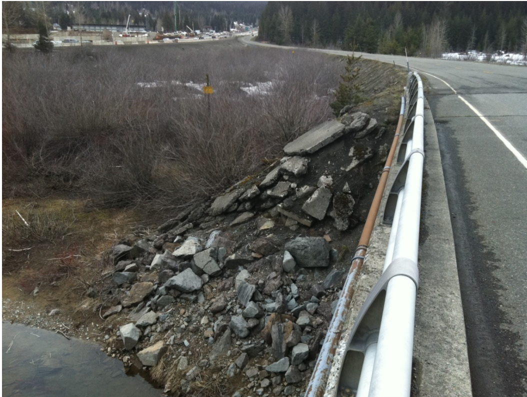
Photograph 2-2 View facing north of west side of USFS Road 4832 and fill embankment. In the background toward the northwest is I-90. May 2011.
