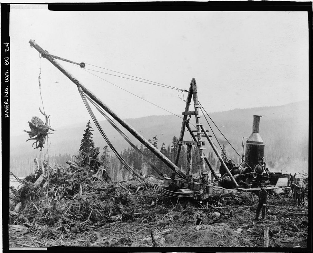
Photograph 3-11 Keechelus Dam Construction, 1913. Stump puller pulling stumps on dam site (USLC, HABS/HAER).
