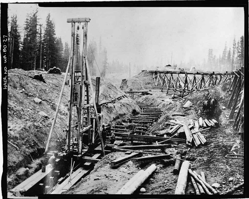
Photograph 3-13 Keechelus Dam Construction, October 1913. Pile driver driving piling for core-wall of dam (USLC, HABS/HAER).
